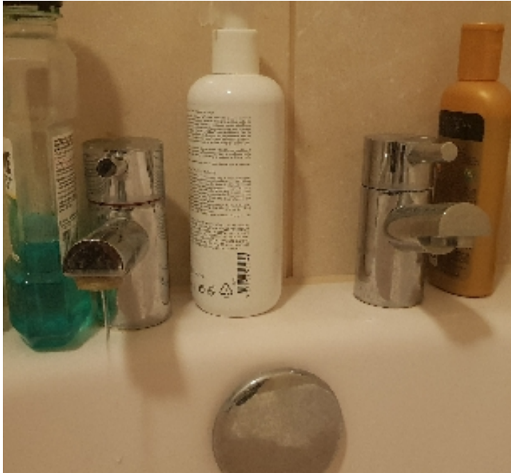
Both taps need to be replaced
