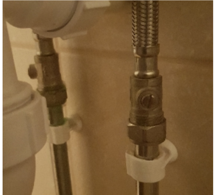
Hot and cold water supply
